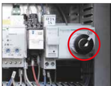
▲ Switch ON/OFF ELCB
